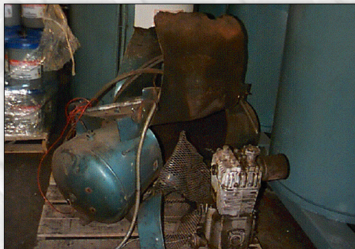
Right view of air tank
