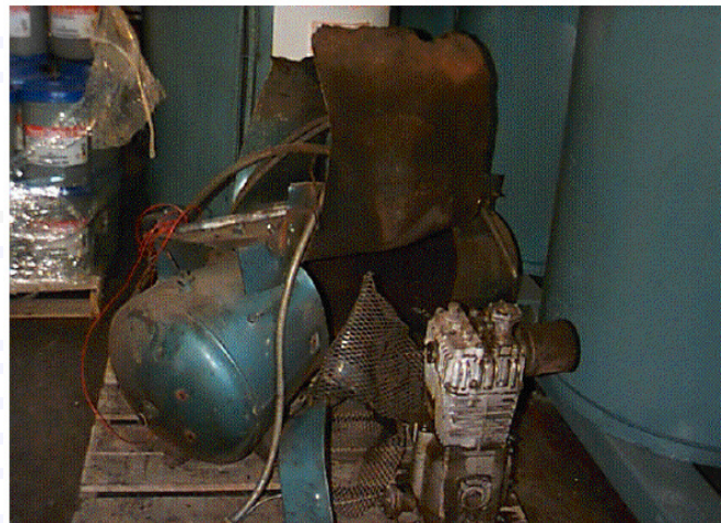
Right side view of the compressed air tank.
